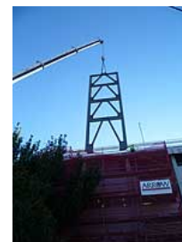
A "k-frame" is lifted into place by crane above block four on the Wellington campus.
