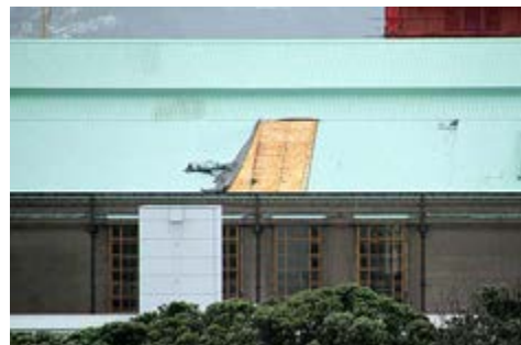
Photos of the Museum Building roof taken by Information Technology Services support analyst Chris Harris.
