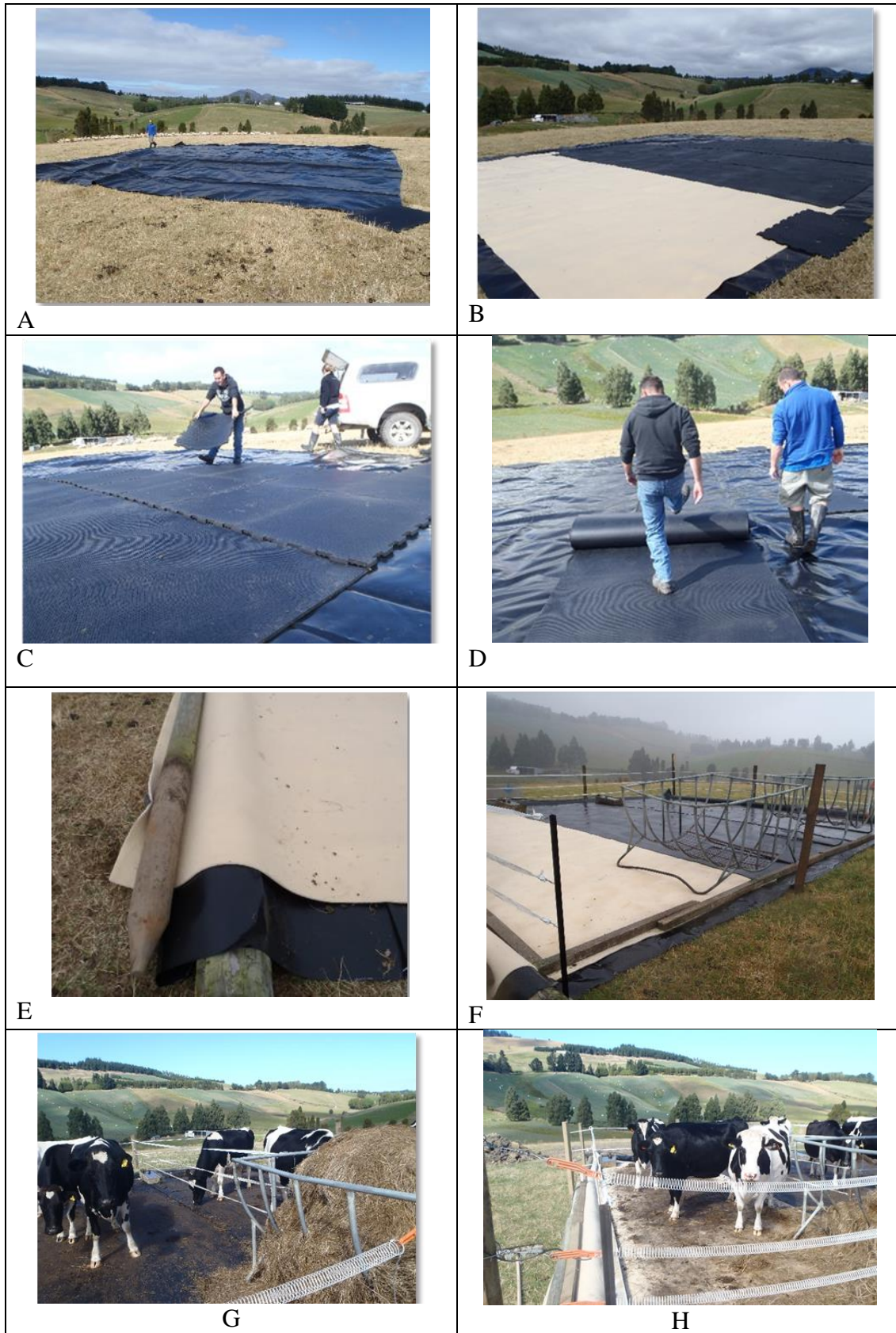
Figure 1. Photos of the portable pad experiment. The geotextile, interlocking mats and rolled rubber surfaces are shown in photos B, C, and D, respectively.
