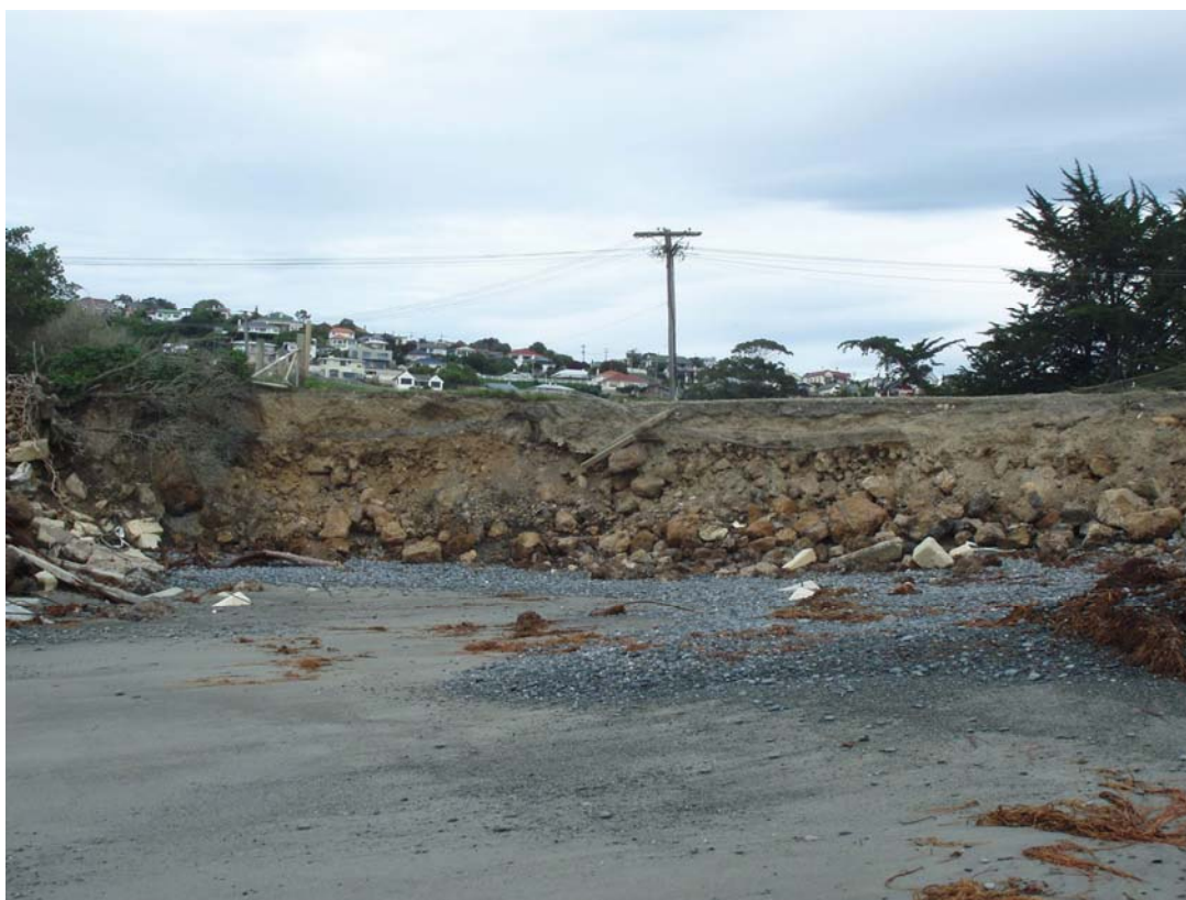
Figure 6: Reclaimed land immediately north of Holmes Wharf exposed by wave attack (the northern abutment of the wharf is at far left). The reclamation consists of unconsolidated rock rubble, masonry, asphalt and soil. Photo 12 March 2009.
