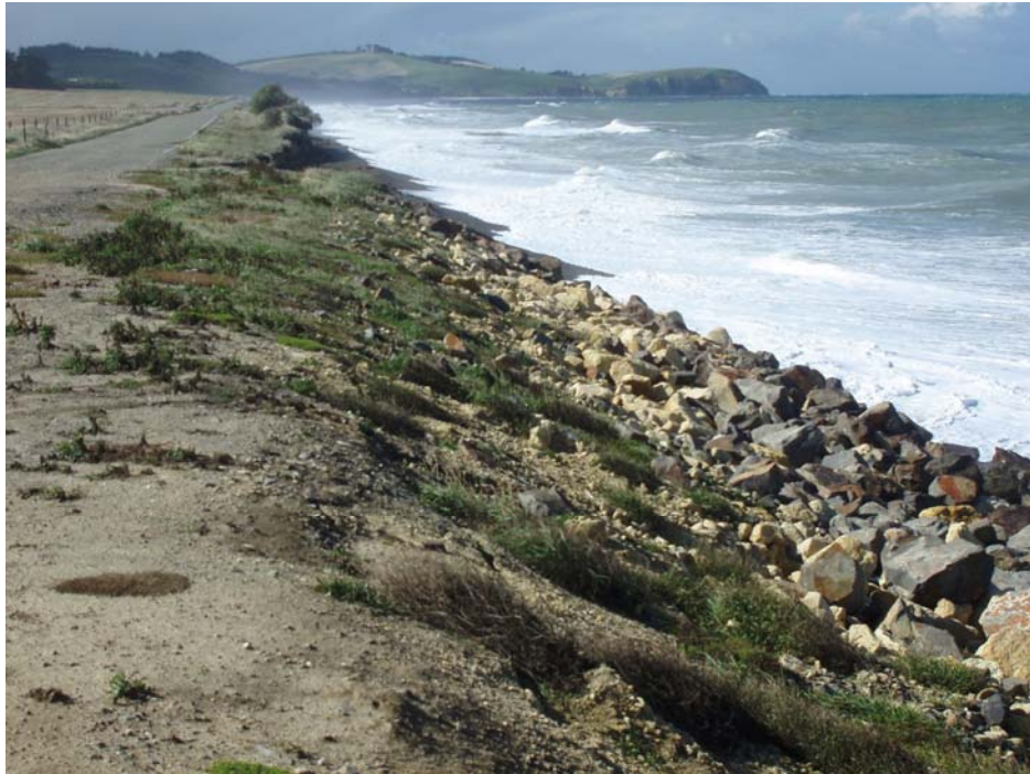
Figure 15: The closed section of Beach Road, near the intersection with Thousand Acre Road, looking north towards Cape Wanbrow. An actively eroding section of cliff can be seen beyond the rock armouring. Photo 11 March 2009.
