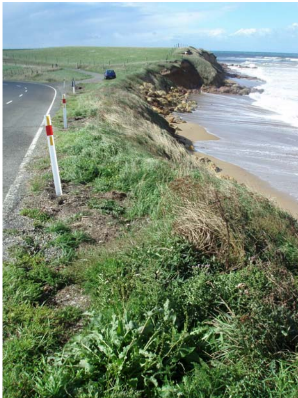
Figure 16: Waianakarua Road – view towards the north from immediately south of Ore Point. The most distant rocks on the beach are natural, but the paler rocks right of the car have been placed to protect the road. In the foreground, the seaward road edge is actively slumping outwards. Photo 11 March 2009.
