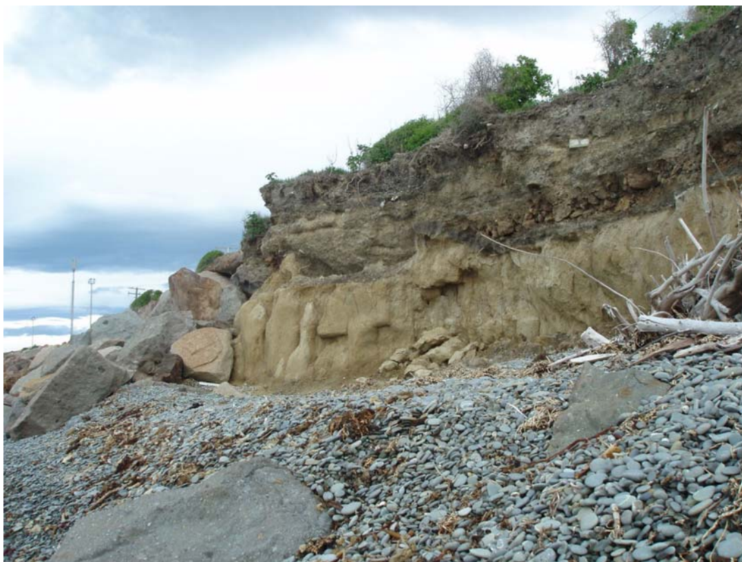
Figure 8: The beach at Orwell St, Oamaru. At left is the northern end of the rock armouring placed to protect the railway line. Loess cliffs centre and right were directly attacked by waves in June 2007 and more recently-fallen material is seen at centre. Above the loess is a significant thickness of material from the last ~ 150 years, containing rubble, wood, concrete, glass and metal. The relationship of the visible storm beach (berm) to the present beach is seen in Figs 9 and 10. Photo 12 March 2009.
