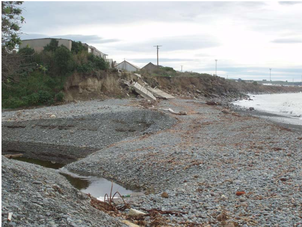
Figure 12: The Pre-cut Joinery factory site near the mouth of Oamaru Creek. Upper photo: Pre-cut Joinery building after undercutting by the sea in 2007 (view towards the south). Rocks in the foreground are part of the rock armouring visible in the lower photo. Photo courtesy of Otago Daily Times, published 2 August 2007. Lower photo: View north from the mouth of Oamaru Creek, towards the Pre-cut Joinery building, in 2009. Fallen concrete slabs from the factory lie across the sea cliff. Beyond is a short section of loess cliffs, and the southern end of the rock armouring placed to protect the railway line. Photo 12 March 2009.
