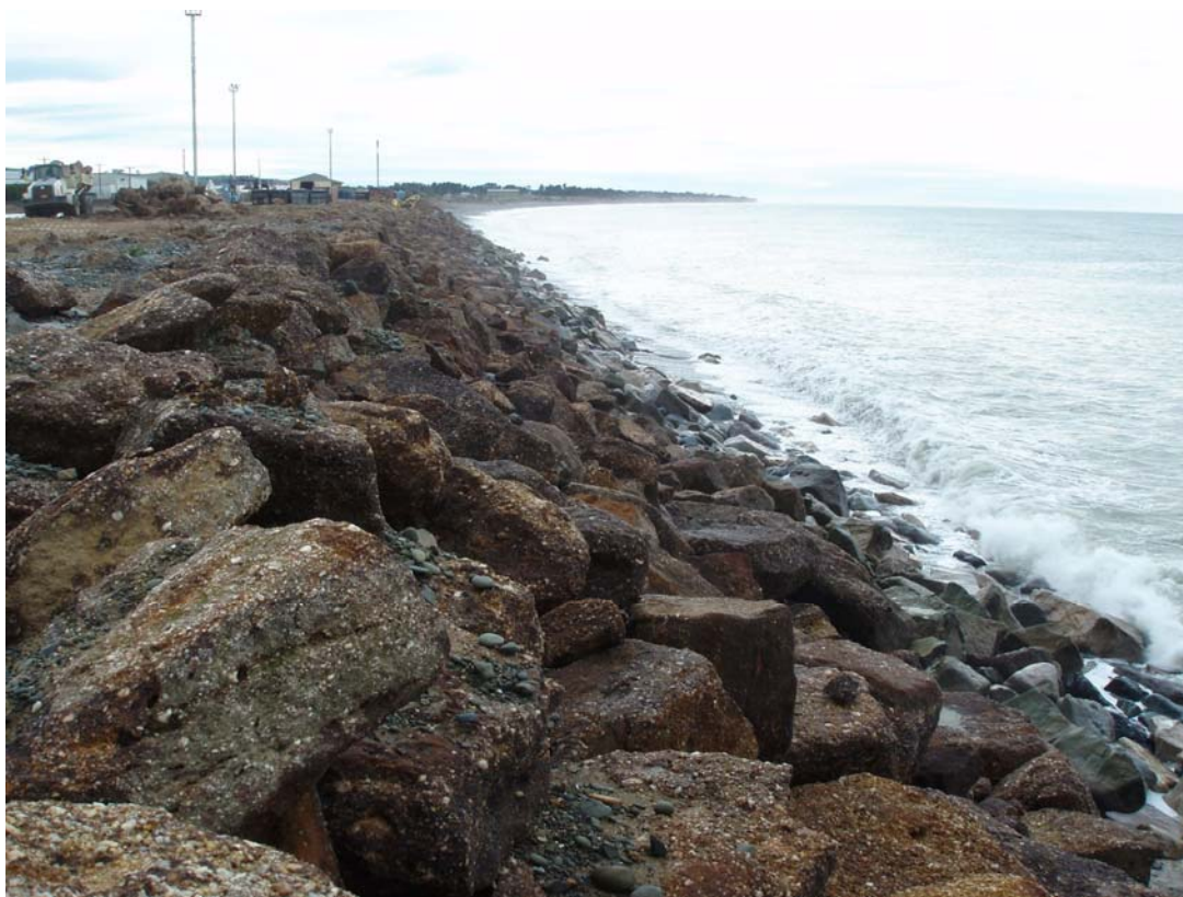
Figure 7: Rock armouring along the coastline at Oamaru Railway Station, looking northeast. The rock wall was undergoing maintenance work at the time of the photo (see yellow digger, just visible upper centre-left). In the distance the cliffed surface of the Waitaki River fan can be seen. Photo 12 March 2009.
