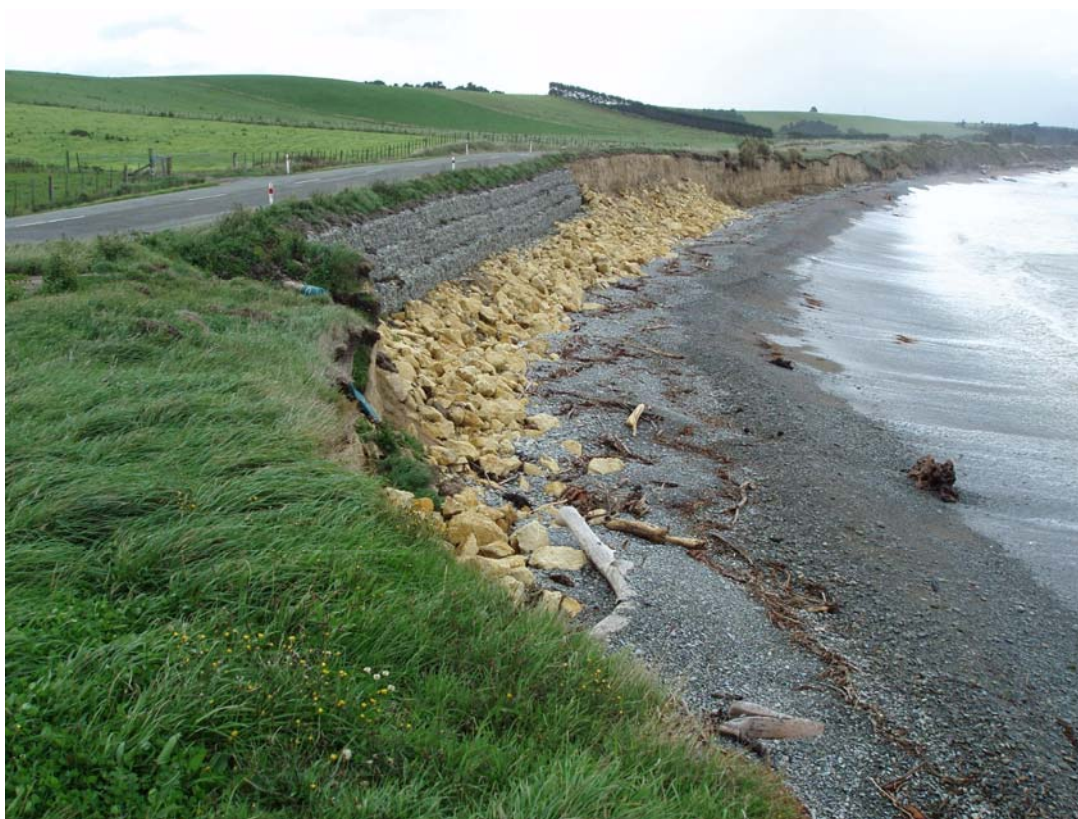
Figure 17: Gabions and rock armouring on Waianakarua Road, just north of the Waianakarua River mouth, looking northwards. Beyond the rock wall, the cliff consists of loess overlying Cenozoic volcanic rocks. Despite this protection work, cracking of the seaward road verge extends to within 60 cm of the road-edge white line. Photo 11 March 2009.
