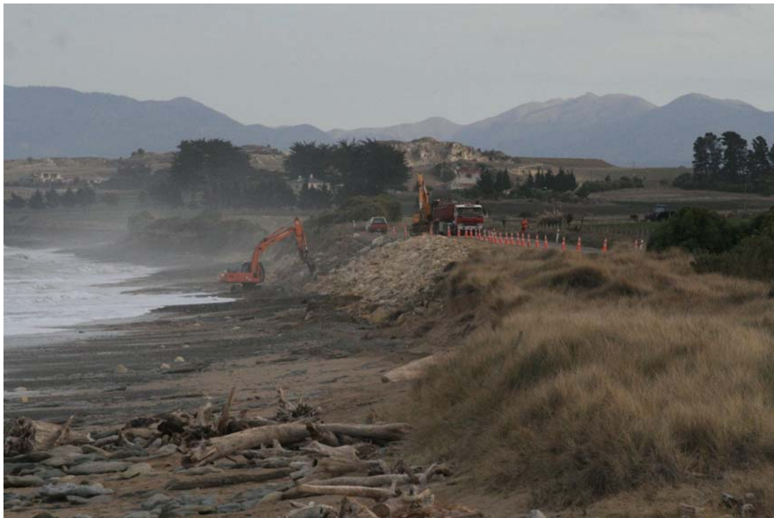
Figure 14: Beach Road near Awamoa Creek. Upper photo: North of Awamoa Creek, part of Beach Road has been shifted inland. In the foreground are materials used in ineffective attempts at cliff protection. Road works just visible in the middle distance are shown in the next photo.
