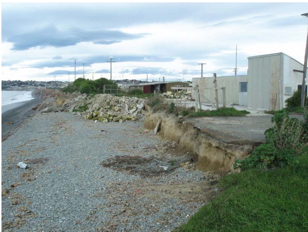
Figure 9: The Firman joinery factory site in Lower Weaver St. Upper photo: The site during a period of active erosion (view towards the north). Note the height of the cliff exposed to wave attack during storm conditions. Photo courtesy of Otago Daily Times, published 27 June 2007.
