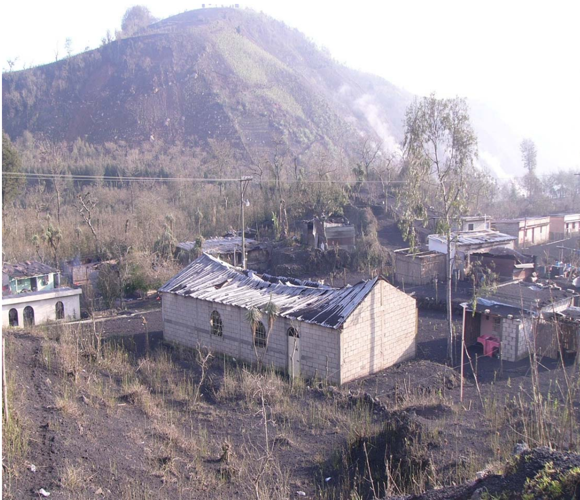
Figure 4.4 Roof collapse due to tephra loading, San Francisco de Sales (photo: Gustavo Chigna, INSIVUMEH).
