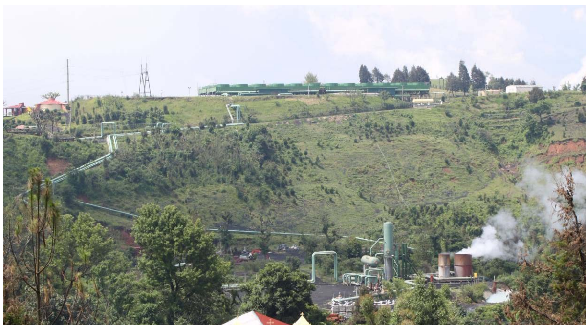
Figure 3.1 Amatitlán geothermal plant.
