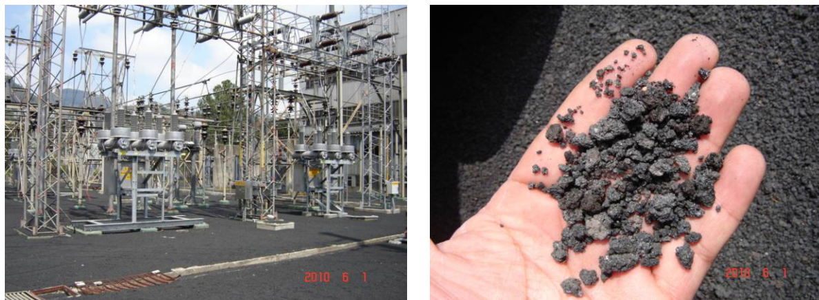
Figure 3.4 Coarse tephra deposited at Laguna substation (see Figure 3.5 for location)(photos: EEGSA)
