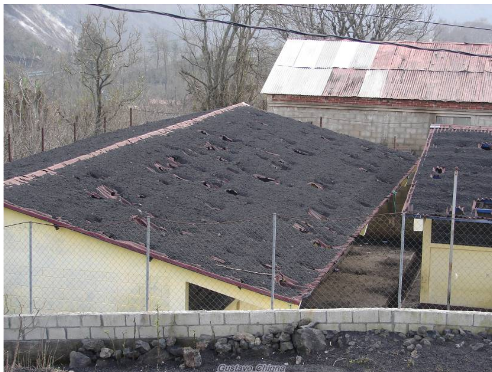
Figure 4.3 Ballistic damage to roof, San Francisco de Sales (located approximately 3 km north of the vent). Ballistics in this area reached 25 cm in diameter (long axis) (photo: Gustavo Chigna, INSIVUMEH).
