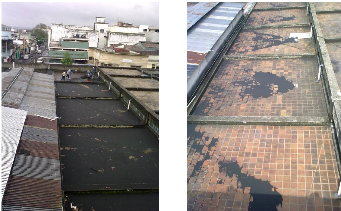
Figure 3.11 Cleanup of tephra from roof in progress (left), and abrasion damage to surface coating on roof (right).
