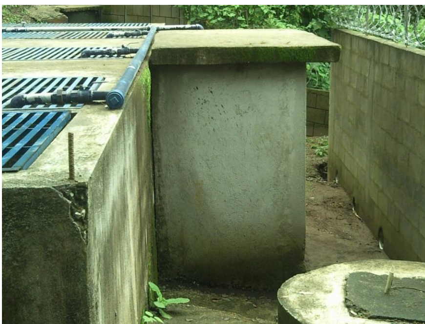
Figure 3.8 Aerobic digestion tank, small-scale wastewater treatment plant serving condominium development (photo: Mapreco).
