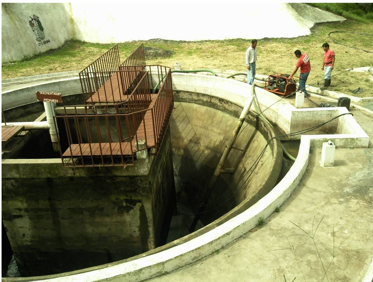
Figure 3.6 Cleaning out Imhoff tank at University of San Carlos, Guatemala City (photo: Mapreco).
