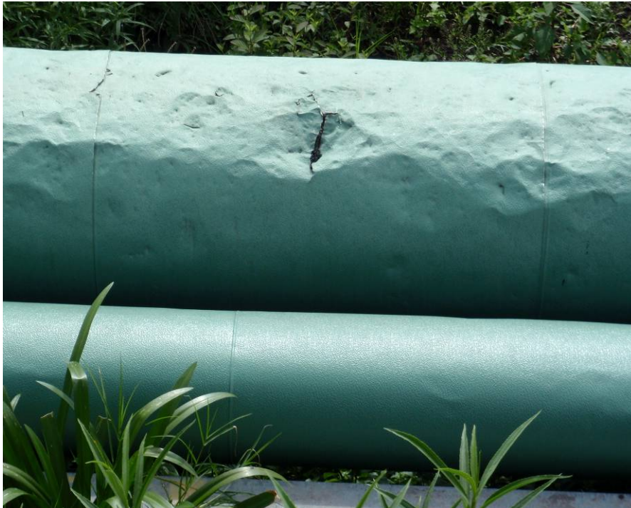
Figure 3.2 Superficially damaged pipe cladding at the Amatitlán geothermal power plant (dent is approximately 20 cm wide).
