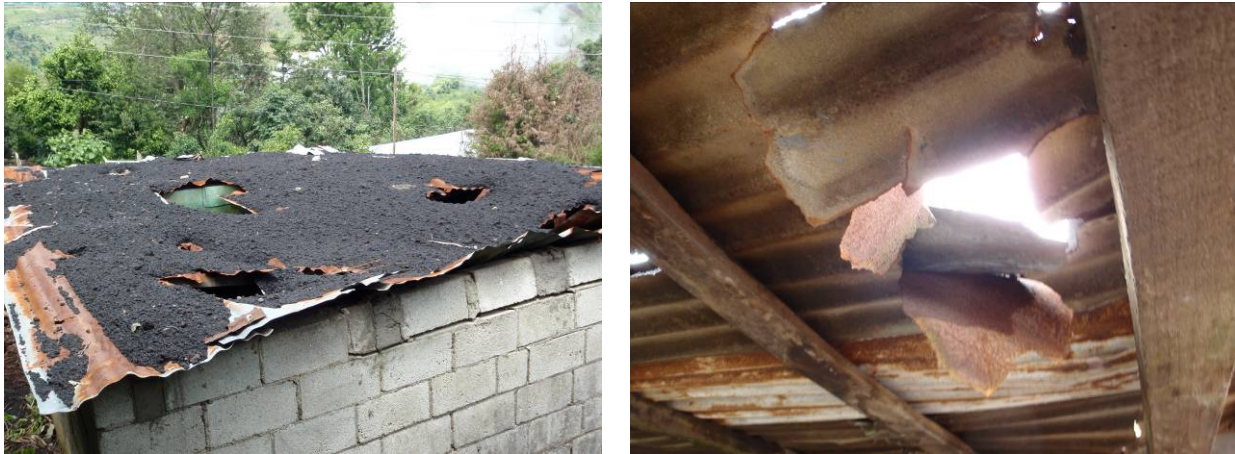
Figure 4.6 Tephra deposition and ballistic damage to roofs, San Francisco de Sales, 19 September 2010.
