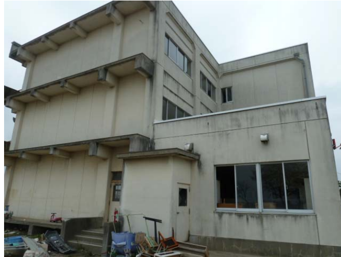
Figure 67 Yuriage Junior High School is constructed on ground which is raised 1.8 m above the surrounding fields. This helped to mitigate damage from the tsunami flow and only contents damage was observed (EEFIT, 2011). 823 people took refuge here.
