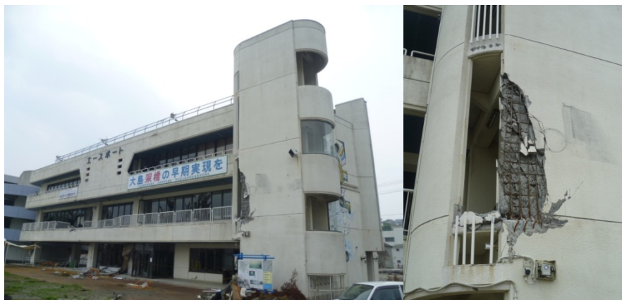
Figure 46 An office building in the inner harbour was unused on March 11 th . This building sustained debris damage to the external stairs (front right) which face the harbour. Minor scour occurred along the seaward face of the building, and around the base of the external stairs.
