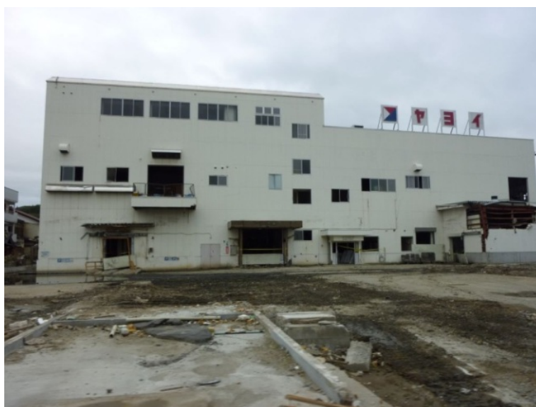
Figure 47 The Yoyoi food factory, where 400 people took refuge. Inundation height was around 8 m here.
