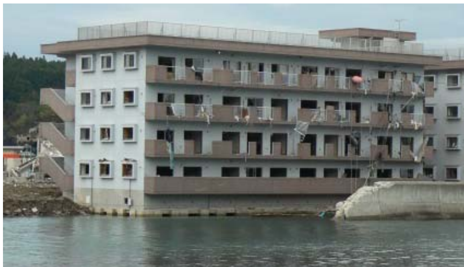
Figure 55 Matsubara apartment block viewed from the seaward side with waterborne debris to the 4 th storey. The low seawall has been destroyed in the tsunami return flow and was sheltered in part by the apartment building. The foundations of this building are exposed above the water level due to extensive scour.
