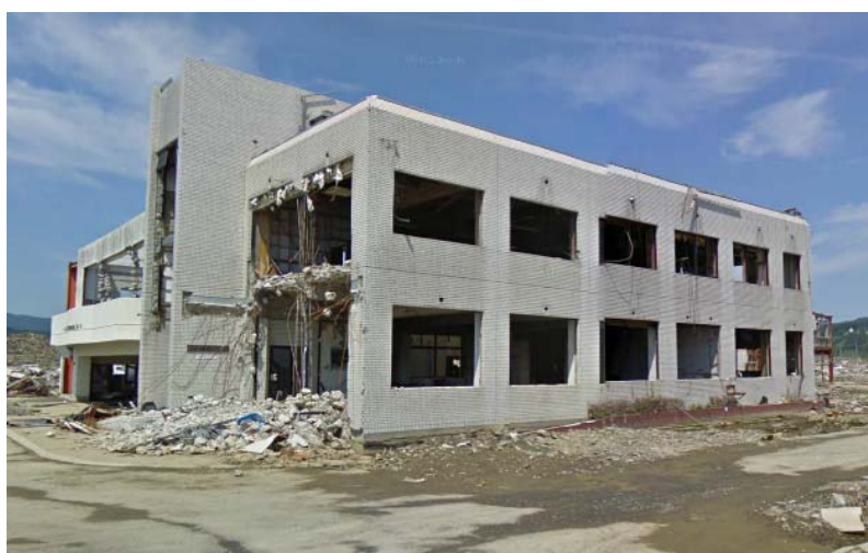
Figure 59 Minami-Sanriku fisheries co-operative building which was overtopped on March 11 th . Image credit: Google Streetview, August 2011.
