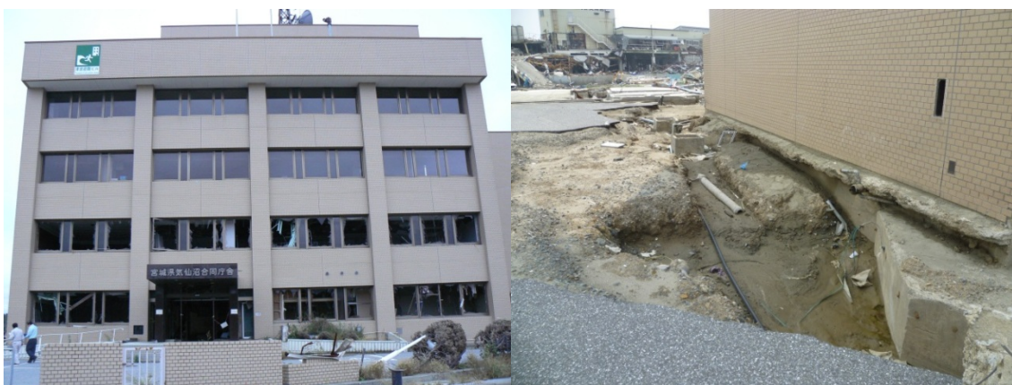
Figure 50 The Prefectural Government offices suffered extensive scour and heavy inundation of 8 m. This building was constructed after 2004 and displays tsunami vertical evacuation signage at roof level. 200 people survived the tsunami in this building
