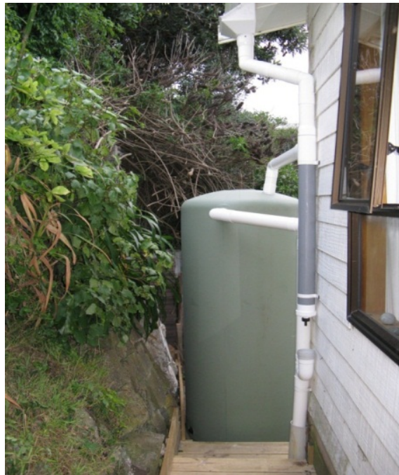
Figure 2 Rainwater tank (1000 litre) with first flush diverter system (grey length of pipe with removable cap for cleaning) (S. Abbott photo).
