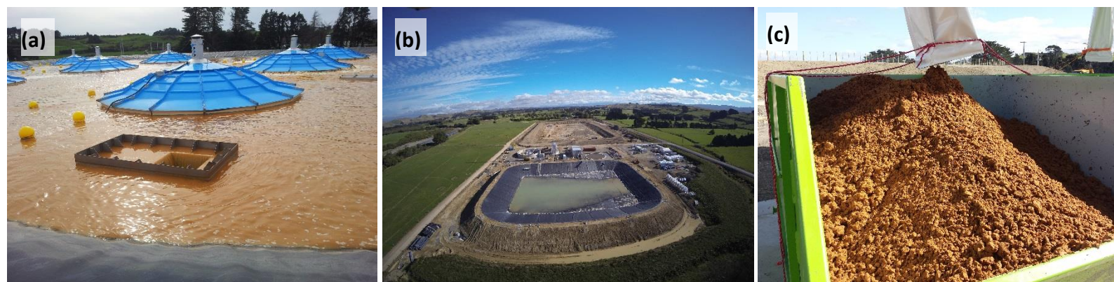
Fig. 2. Examples of aerated biological treatment and treatment bio-solids export at Fonterra Pahiatua site: (a) aerated treatment pond, (b) 100,000 m 3 storage pond and (c) treatment bio-solids export to composting plant.
