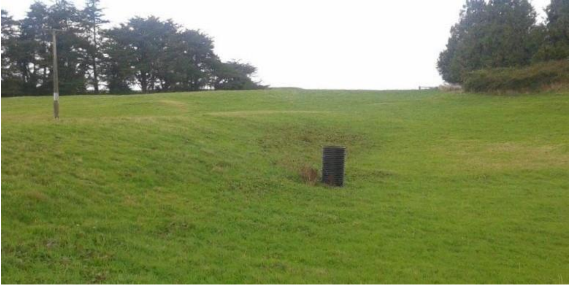
Figure 2: Photo of an upstand riser installed in the ponding area of a detainment bund. The riser is connected to an outlet pipe that passes through the bund, which discharges ponded runoff on the downstream side.
