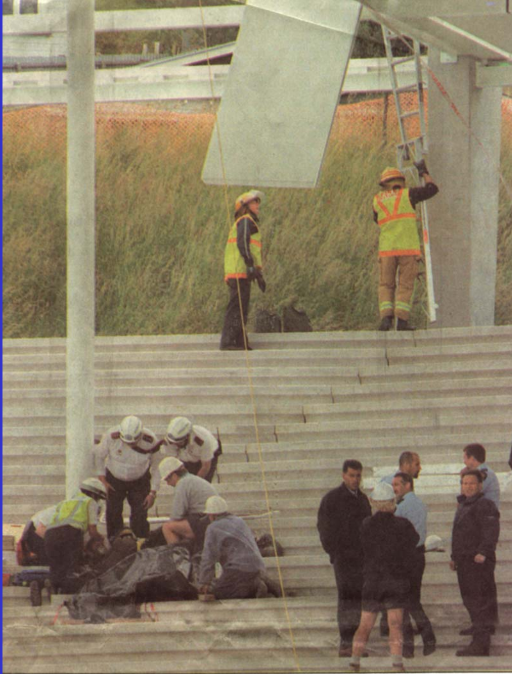
Ambulance staff tend to the injured man after yesterday's fatal accident at Carisbrook. In the background, firefighters inspect the roofing panel which collapsed, sending two men plummeting to the ground.
